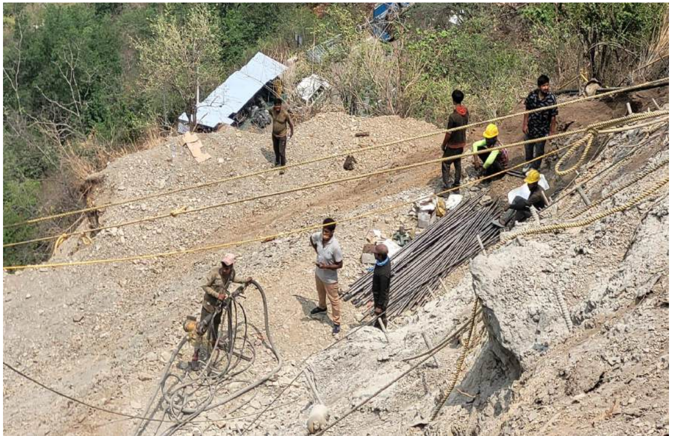
Installation of Self driven anchors (SDA-32mm dia & 13M long @2M C/C Bothways)
