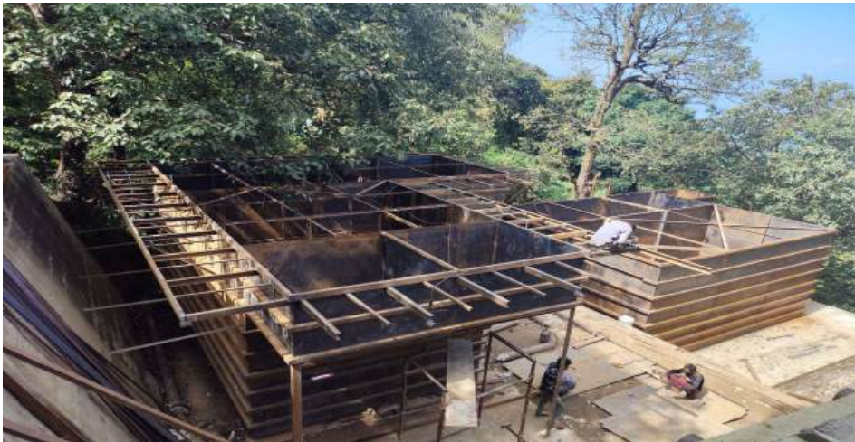
Company Gardan STP 0.70 MLD
